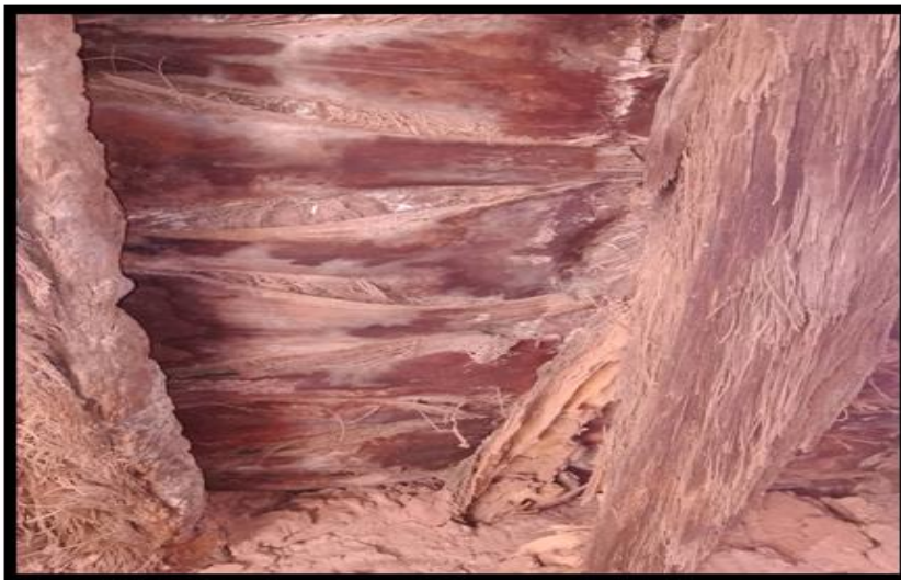
Figure No. 07: Represents termites. Figure No. 08: Represents wood damaged by termites.
