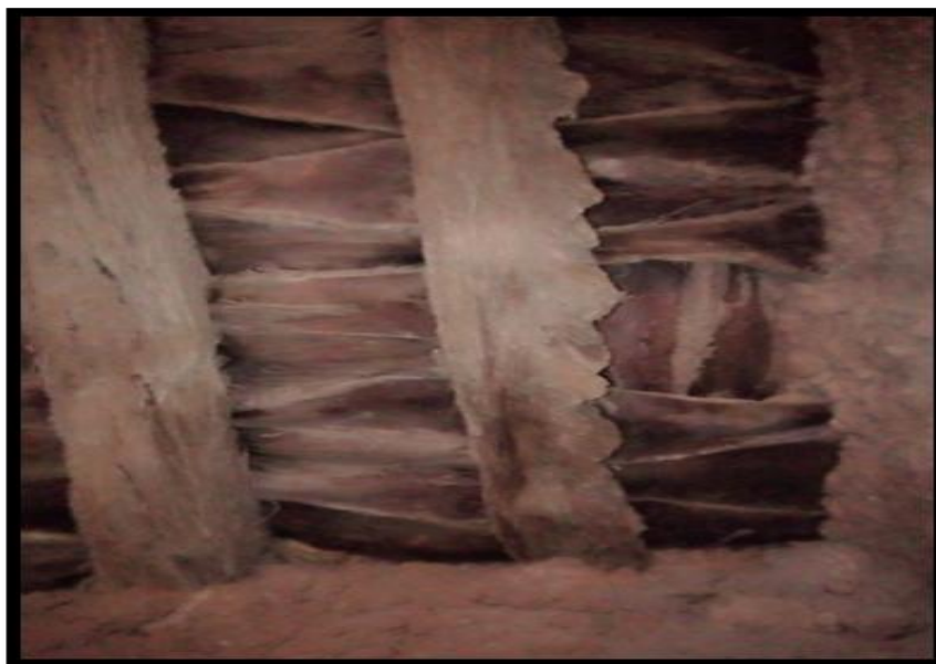
Figure No. 03: The Process of Roofing Using Wood and Palm Frond Bases
